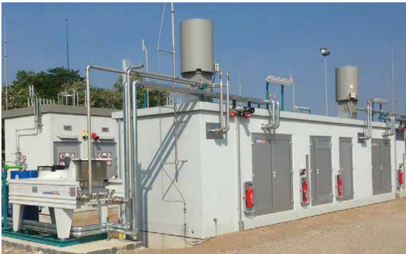
VPT TURN KEY CONCRETE STATION
