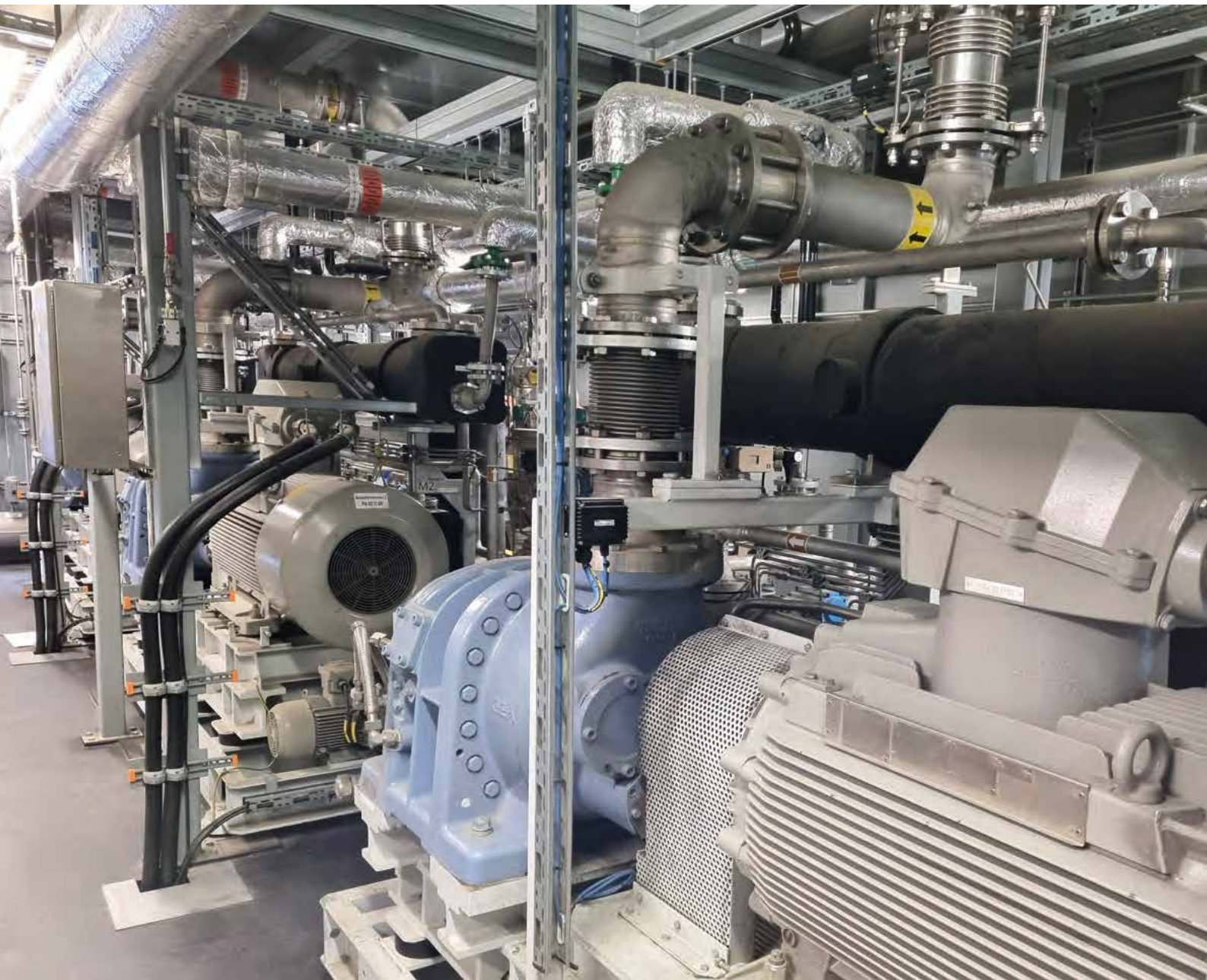
VPT NATURAL & BIOGAS DISTRIBUTION STATION
