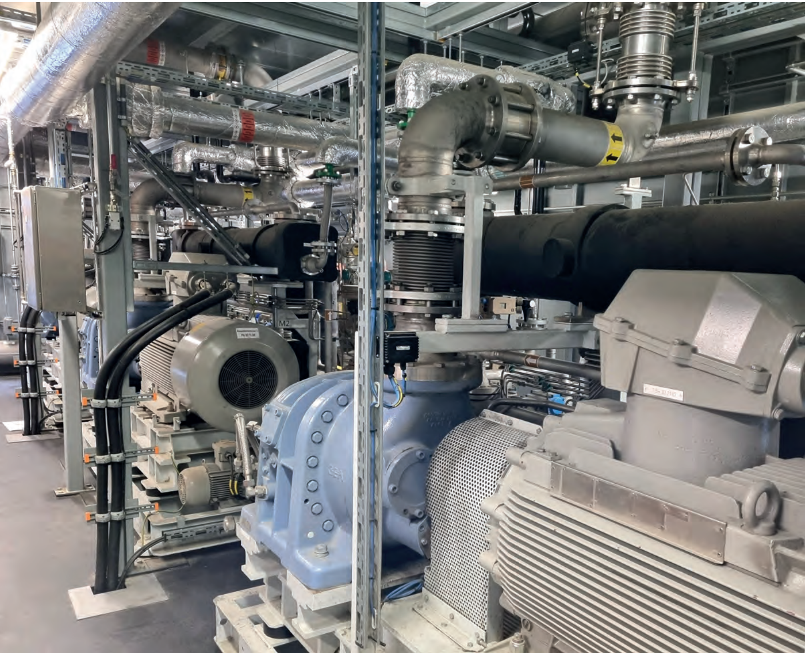
VPT NATURAL & BIOGAS DISTRIBUTION STATION
